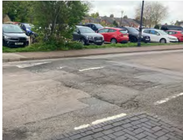
Figure 30: A well-worn road hump.
