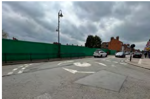
Figure 32: Low quality, well-worn road surfacing and markings at the roundabout of Church Street and Radcliffe Street.
